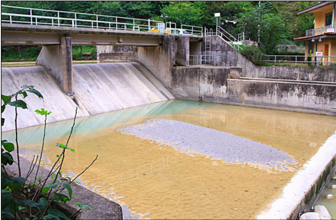
Figure 6: Sardabroud micro hydro power plant.
