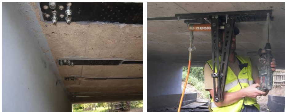
Figure 6: Steel anchorages bolted to bottom surface (left); stretching device on site (right)
