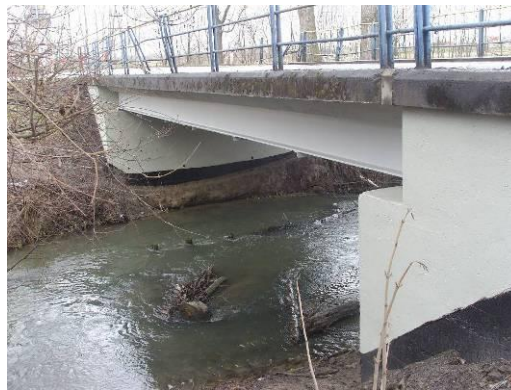
Figure 7: The steel – concrete before rehabilitation
