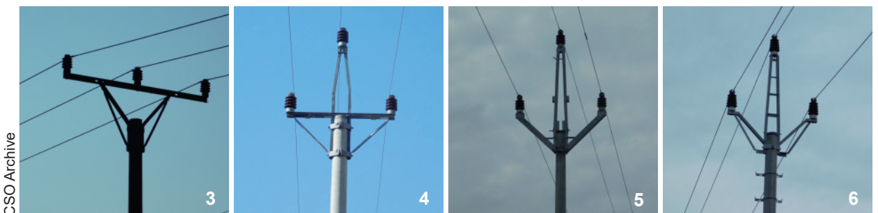
Fig. 3–6. Four basic cross-arm types used for medium-voltage electrical lines in the Czech Republic: a horizontal console with upright insulators (“killer pylon”; 3), Delta (4), Pařát (5) and Delta variant (6).
