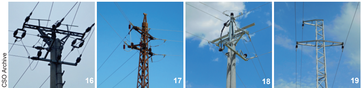
Fig. 16–19. A concrete branch pylon with three horizontal cross-arms, upper, lower and crosswise jumpers and two benches (16), a steel branch pylon with two horizontal cross-arms (17), on which extremely high mortality was found. It was replaced with the pylon in Fig. 18; a concrete pylon with Pařát and horizontal cross-arms and more bird-protection measures: a horizontal plastic element as a safe perch, a jumper insulation and perch discouragers on the horizontal cross-arm (18); a steel pylon with two cable levels and suspended insulators (19).
