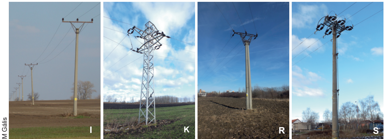
Fig. 5. Basic categorization of 22 kV pole configurations in study area: (I) utility poles in straight line direction, (K) branch pole with cross-arms and different combination of pin-insulators and jumper wire locations, (R) corner pole with different combination of jumper wires location, (S) powerline switch disconnector and (T) electric pole transformer.
