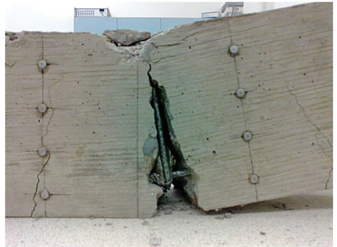
Fig. 15 Failure of the beam containing 50% FEG.
