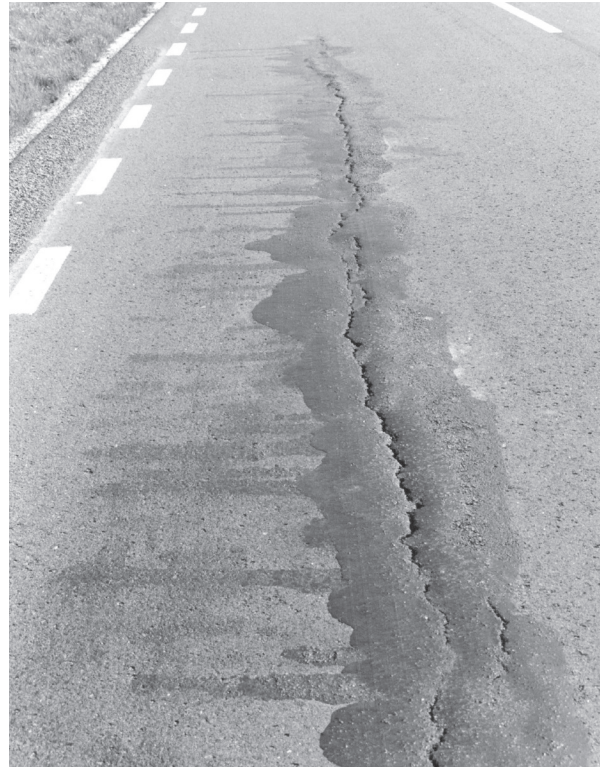
Figure 1: Longitudinal crack in the surface as a result of uneven settlement of the embankment.
