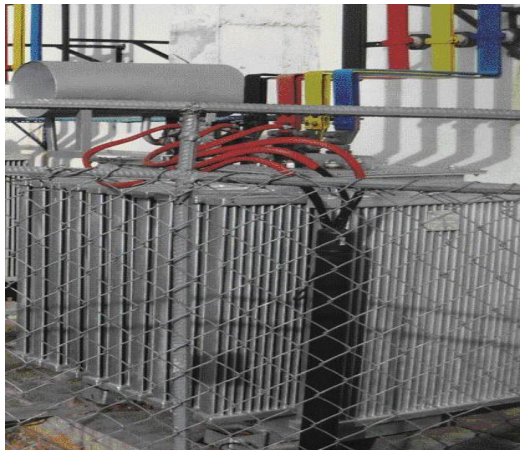
Figure 7. The investigated transformer.
