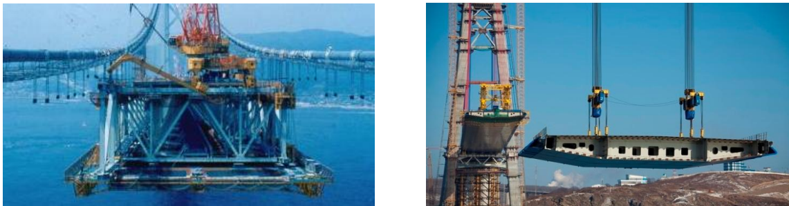
Figure 1. The longest suspension and cable stayed bridges today: Akashi Kaikyo (left) and Russkij (right)
