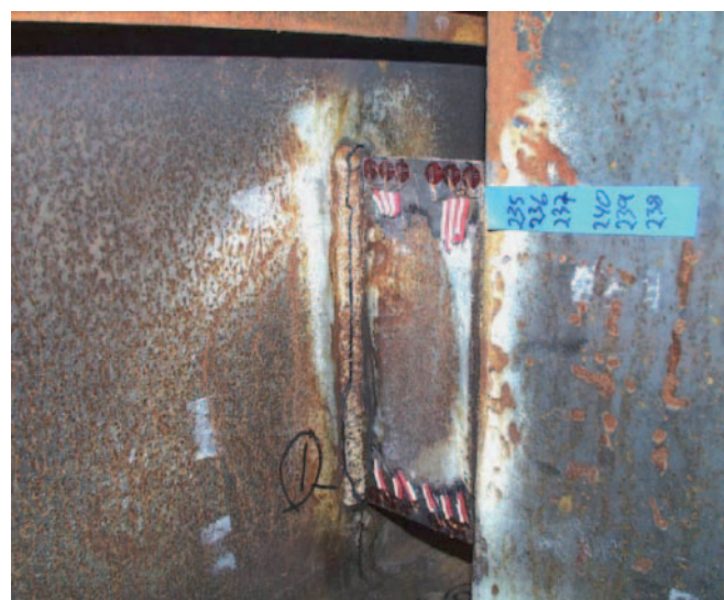
Fig. 5. Example of fatigue crack in welded joint of ship structure detail [6]
