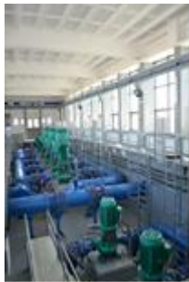
Photo 1. The Chirița pumping station
