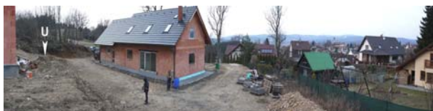
Fig. 2. Panoramic photo of the building site studied, 26 March 2015. House #1 is in the middle; corner of the House #2 is on the left side. On the right is a view of the Jablonec city. Uranium vein outcrop (indicated by white arrow) is placed on the ramp between both the houses. Photo by Jakub Plášil, with permission of House #1 owner.
