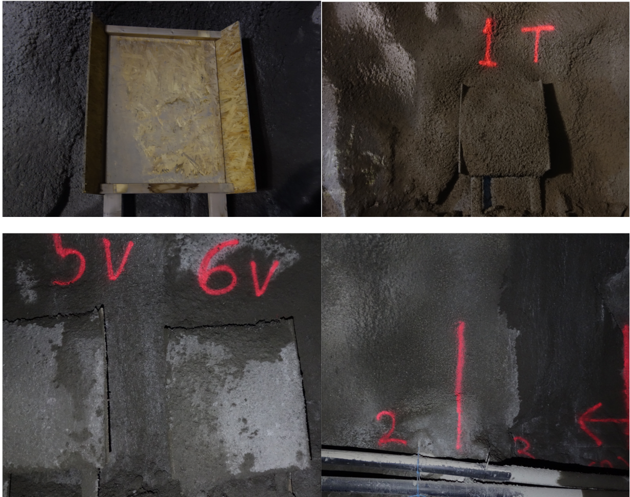
Figure 3 - From top to bottom, left to right i) mould for test samples, ii) marking after finished spraying, iii) drying process and iv) shotcrete sprayed on rock for bond test and extent of wet area at the third section.
