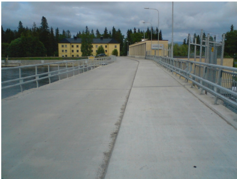
Figure 3 - Non-cracked pavement performed in 2010 in Bodforsens hydro power plant, Boden Un-reinforced and steel fibre reinforced areas in full scale tests. (photo by J. Carlswärd).
