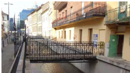
Figure 3. Iron bridge (wrought iron railing and gate, rust eaten steel beam stiffened with a pipe at the bottom) and balconies over the Mill-Channel in Cluj-Napoca
