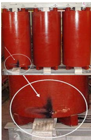
Fig.3. Analysed power transformer with defect of the coil of phase A.
