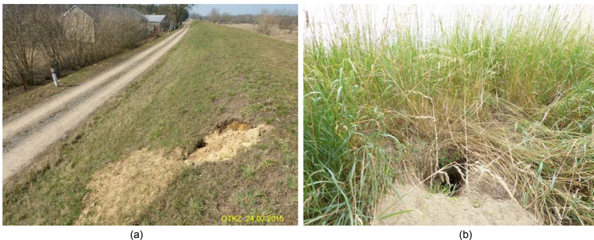
Figure 1. Presents damaged flood banks caused by animals. The holes were caused by the beavers living in the area. Grazing animals on the levees and in their immediate vicinity violates the construction of levees and causes changes in soil mass. Photo by Janusz Orzepowski
