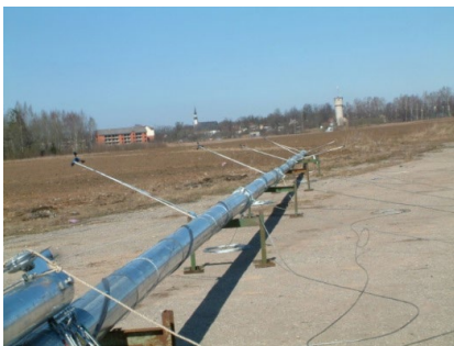
Fig. 5. Installation of the 60-m high mast with a measuring complex Symphonie 9200 together with sensors on metal 1.8-m long mounting boom (site 2).
