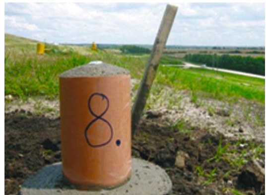
Figure 5. Settlement measuring point.
