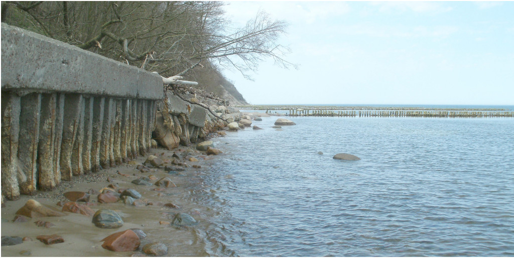
Fig. 10. Damaged shore protection structures west of Svetlogorsk (near the Otradnoye village), 900 m long, built in 1966
