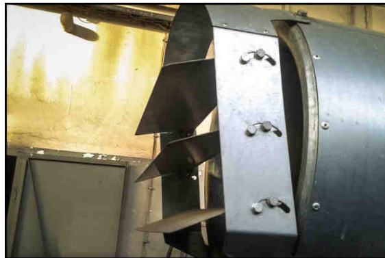
Fig. 8. Jet fan used for the tests and its guide vanes
