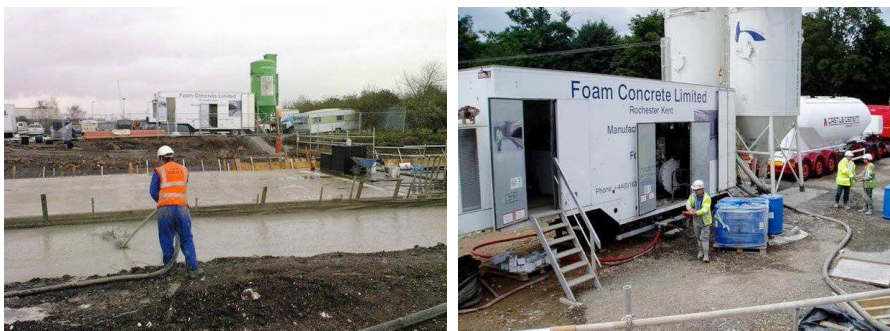
Fig. 3: Figure 1 Pumping foam concrete and the mobile device to produce a mixture [4].
