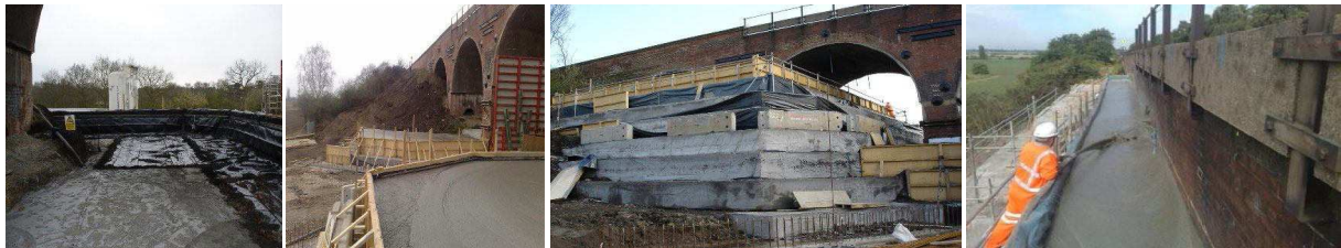
Fig. 2: Views of preparation of the underlay, a poured layer of foam concrete, the pyramidal formwork and application of the last layer of foam concrete.
