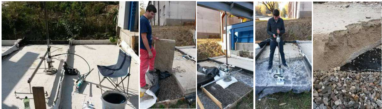
Fig. 12: Views of measurement SLT surface Poroflow 17-5, the removal of the structural system, SLT measurement and dynamic test equipment LDD 100 to the drainage layer.
