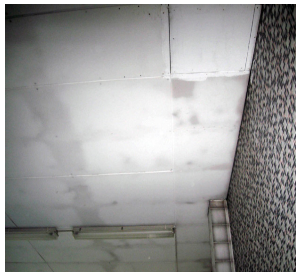
Figure 2 Asbestos boards on the ceiling of the Zasavje swimming pool facility where the patient worked in the 1970s
